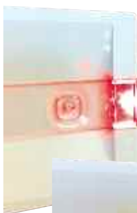
Red warning LED: BATTERY MALFUNCTION
